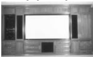
Were these properly measured and equalized after installation? I'll bet they weren't!
